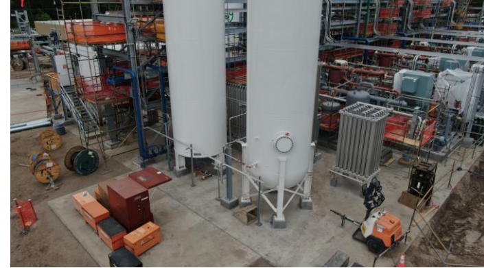
45 TPD plant, Woodbine, GA
