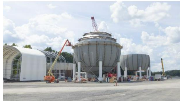
45 TPD Plant, Project Gateway, WNY STAMP, Genesee County, NY
