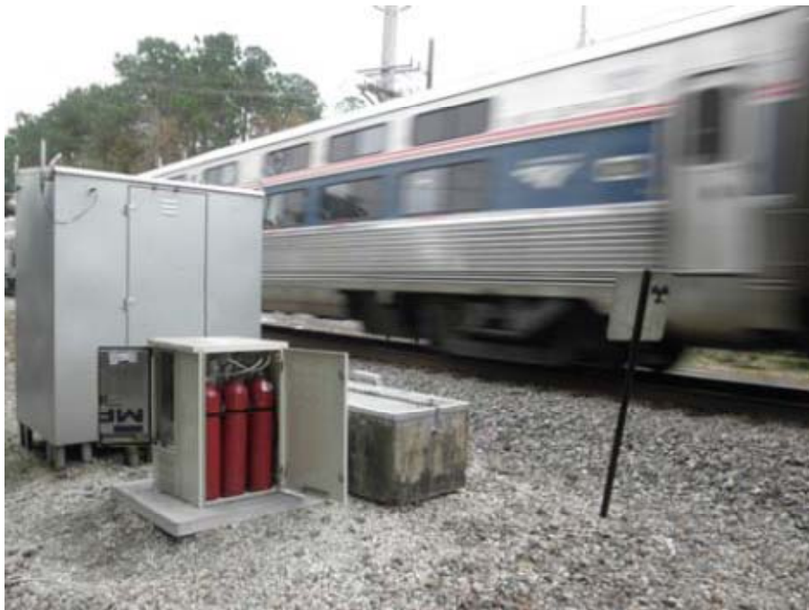
First RR fuel cell deployment at Collins Rd. Jacksonville, Fl.
