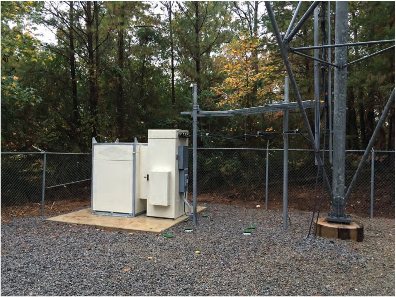
Plug Power's one-pad, space-saving integrated OSP solution.
